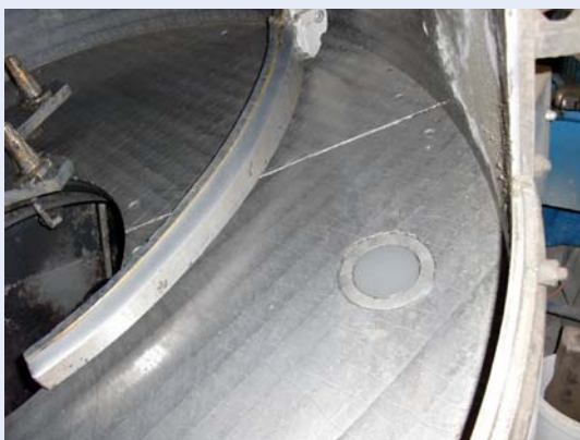
Probe installation in a rotating mixer floor
